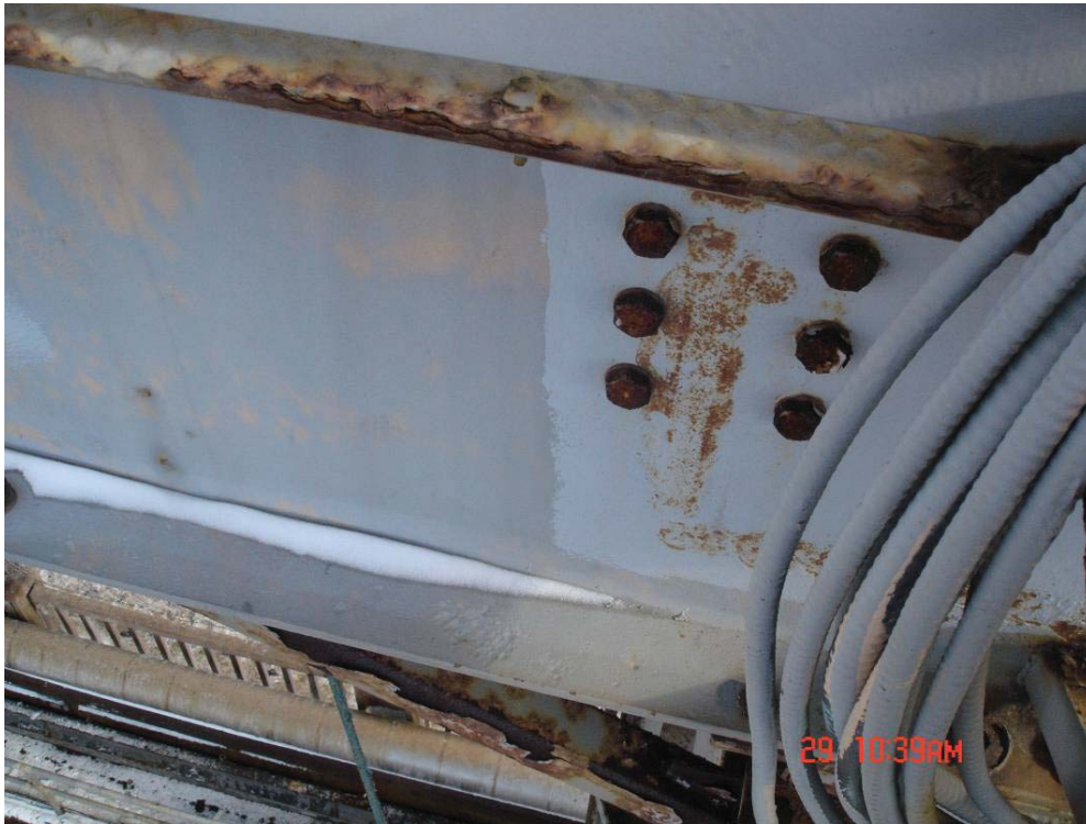
Photo 13 – Surface Corrosion on Connection Bolts for Recent Installation of Beams to Replace Box Beam
