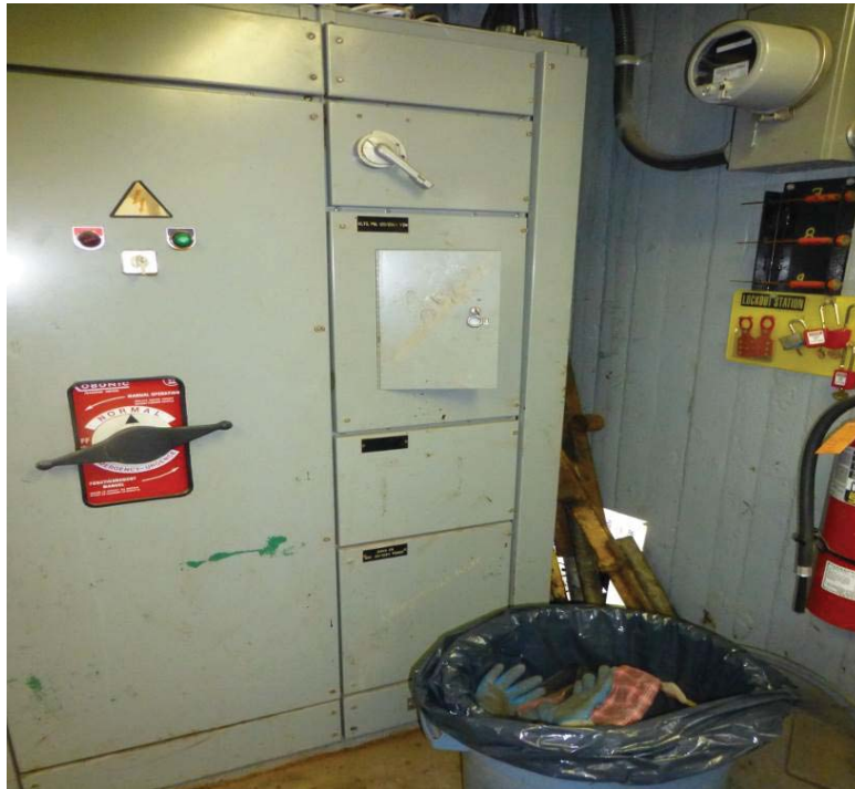
Photo 25 – Existing MCC Transformer, Panel and Transfer Switch
