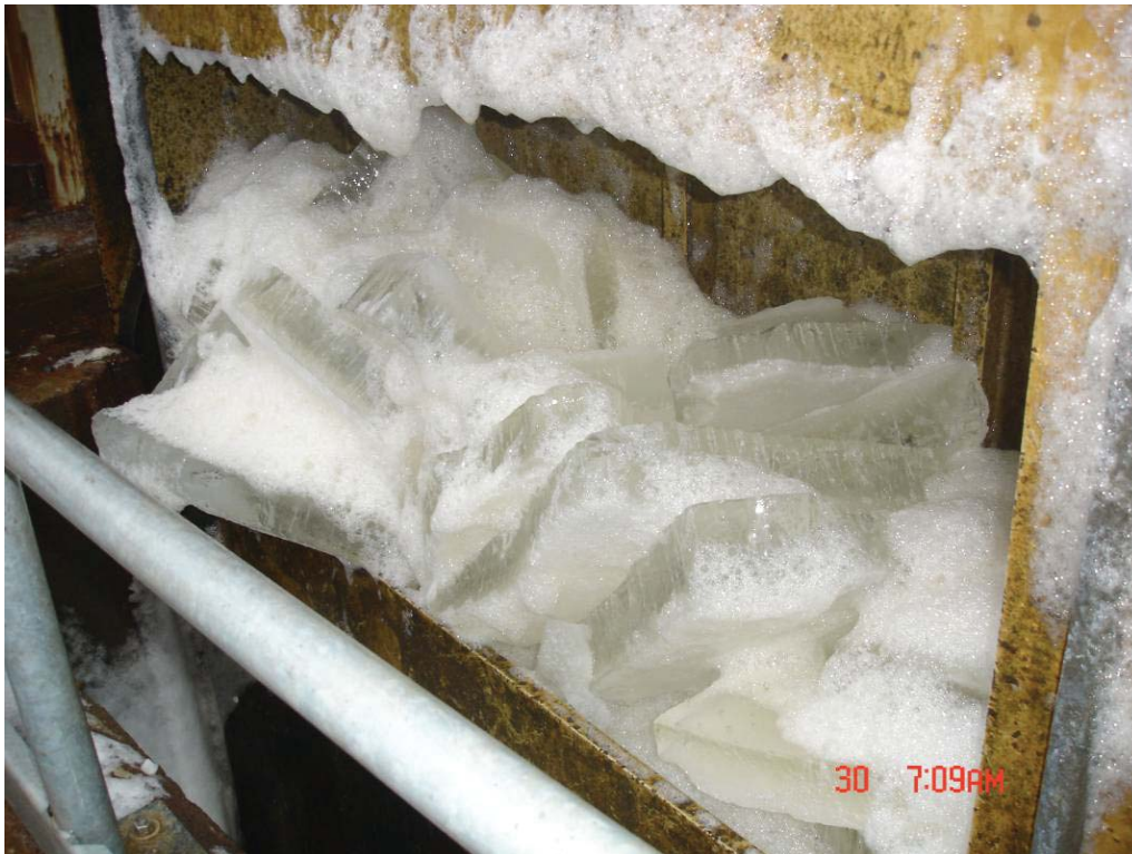
Photo 22 – Ice Collected in Back of Spillway Gate When Opened
