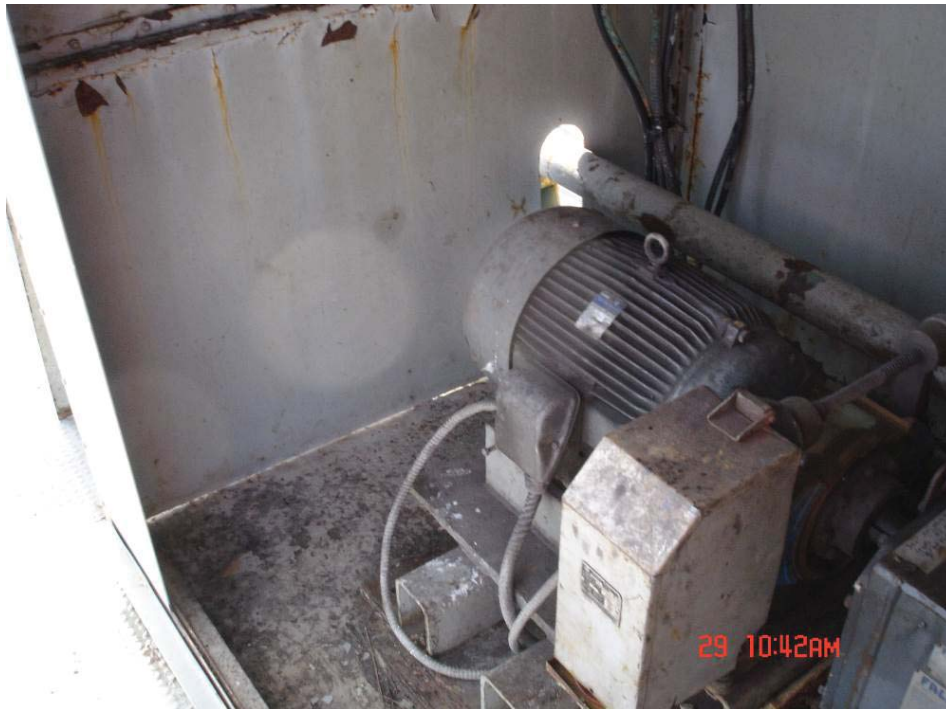
Photo 11 – Perigrip Brake on the Front Side of the Hoist Motor
