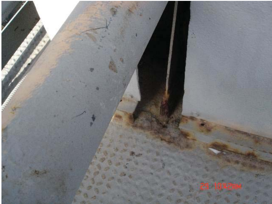
Photo 19 – Drive Shaft Enclosure Penetration Corrosion
