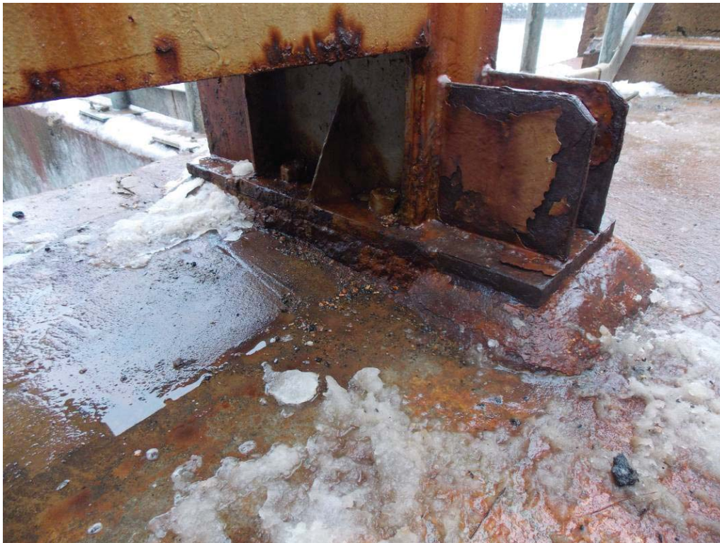
Photo 18 – End Tower Base Plate Surface Corrosion
