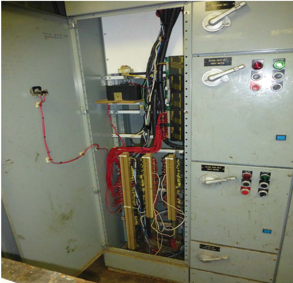
Photo 29: Sluiceway Remote PLC in MCC
