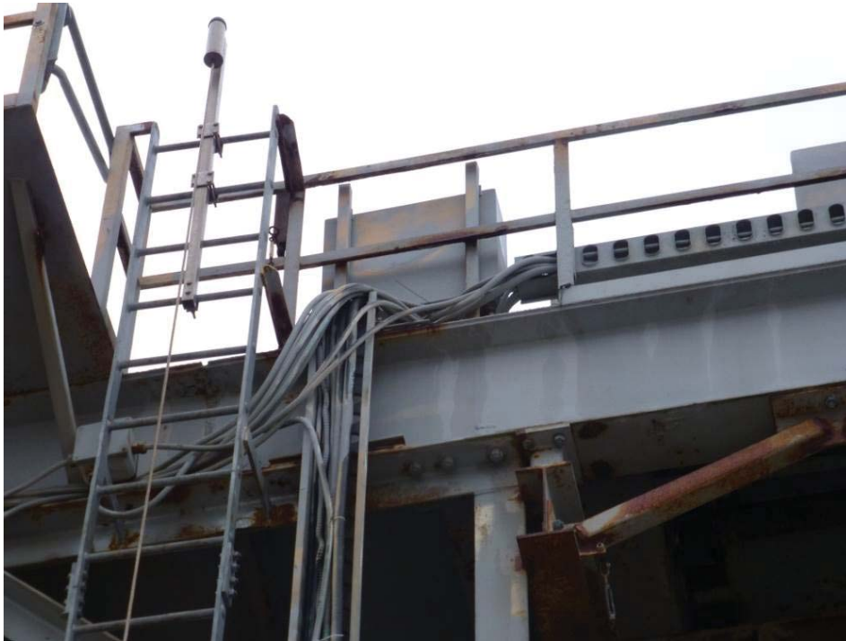
Photo 26 – Gate Structure Cabling
