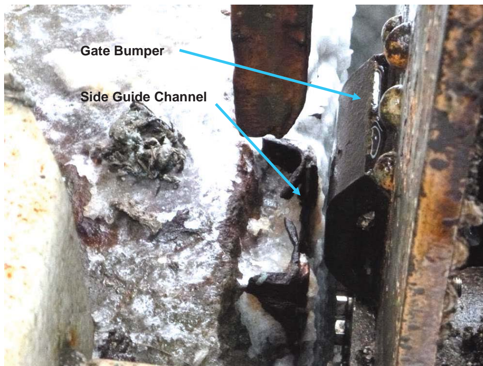
Photo 7 – Deterioration of Embedded Side Guide Roller Path Channel
