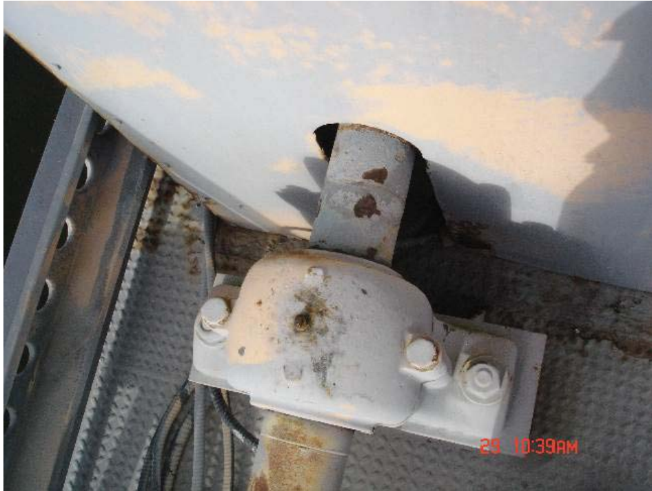
Photo 18 – Drive Shaft Enclosure Penetration
