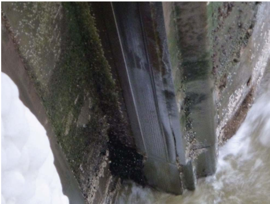
Photo 8 – Deformation of \frac{1}{4} " Roller Path above Lintel (Tidal Side)
