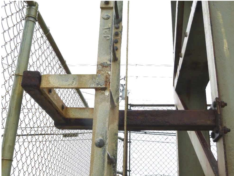
Photo 4 – L-Shaped End Tower Ladder Support Brackets
