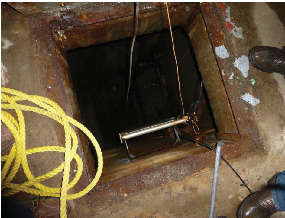
Photo 27 – Head Pond Level Transmitter
