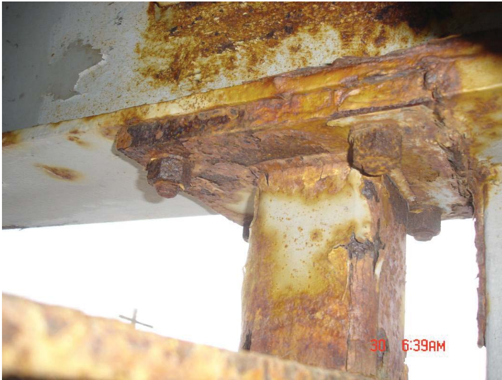
Photo 21 – Corrosion of Hanger Connection for Upper Sheave Support Structure
