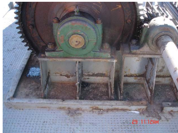
Photo 21 – Drum Enclosure Internal Corrosion
