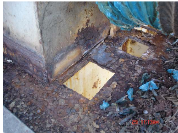
Photo 22 – Drum Enclosure Severe Deck Corrosion
