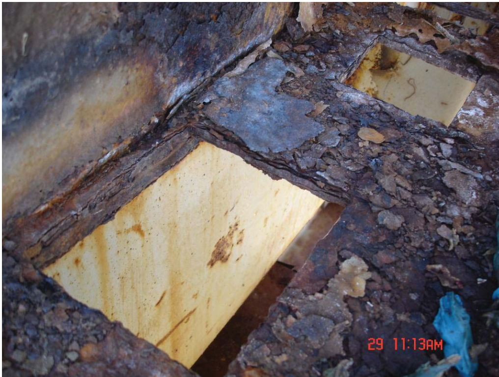
Photo 16 – Floor Plate Corrosion under Drum
