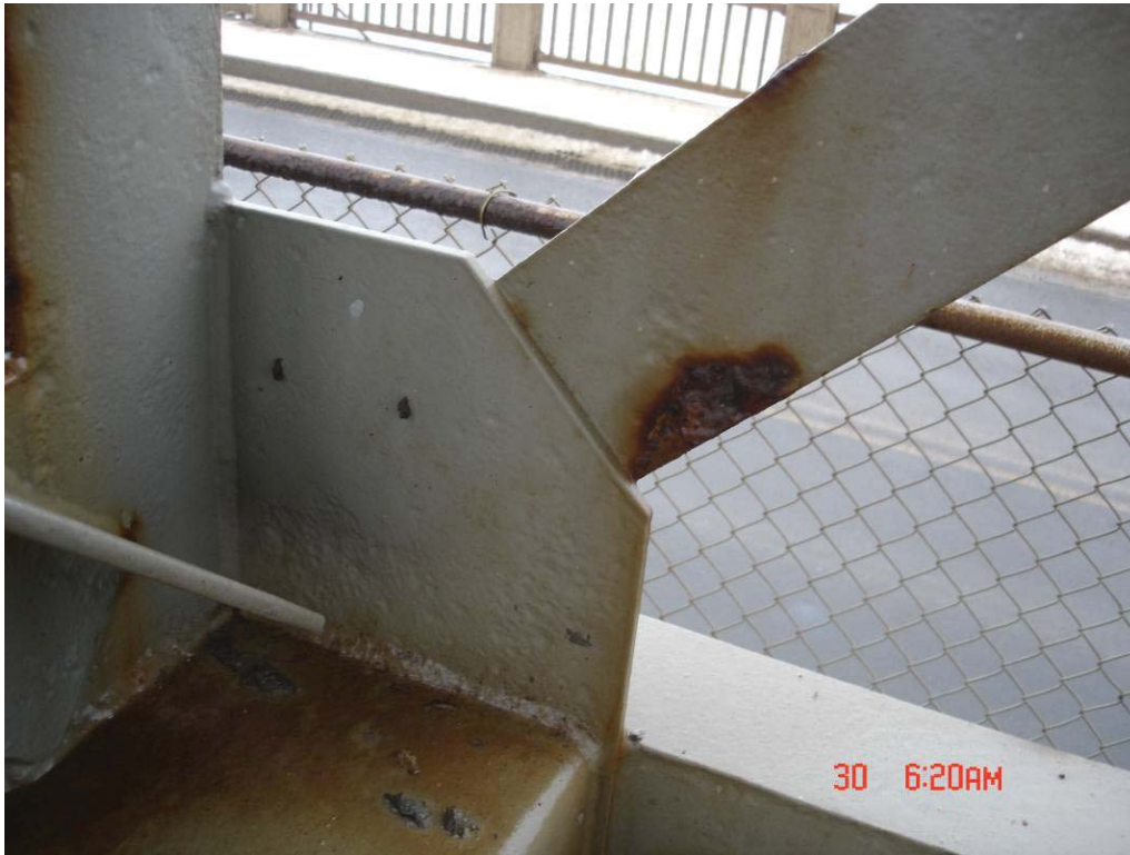
Photo 19 – Hoist Superstructure Typical Localized Surface Corrosion and Staining
