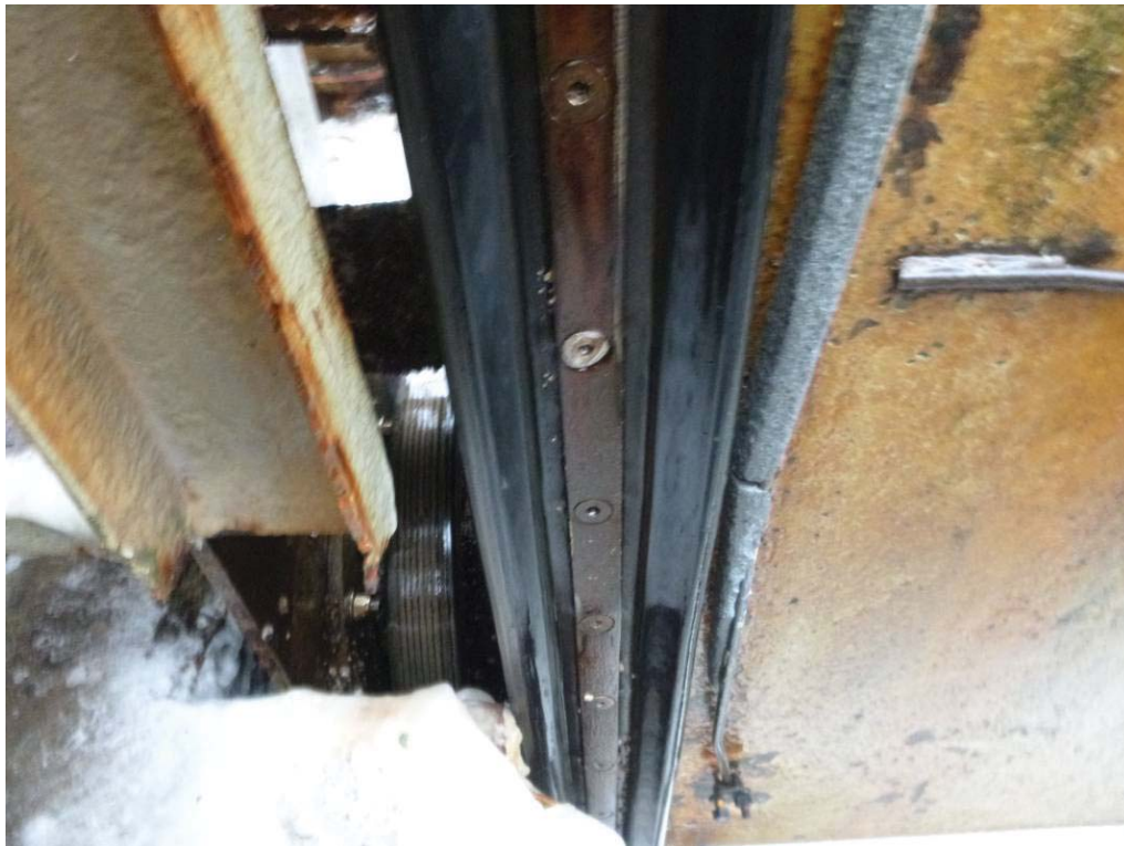
Photo 10 – Partially Twisted Lower Gate Seal and Bent Zinc Anode Adjacent
