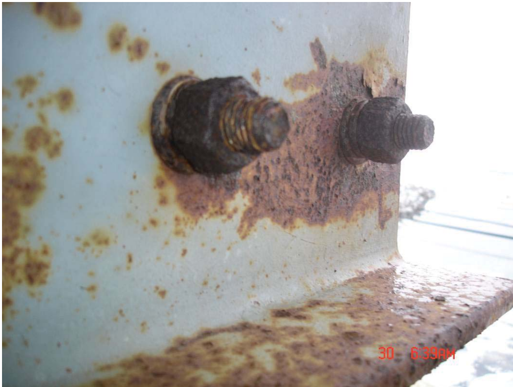
Photo 20 – Structural Bolt Corrosion
