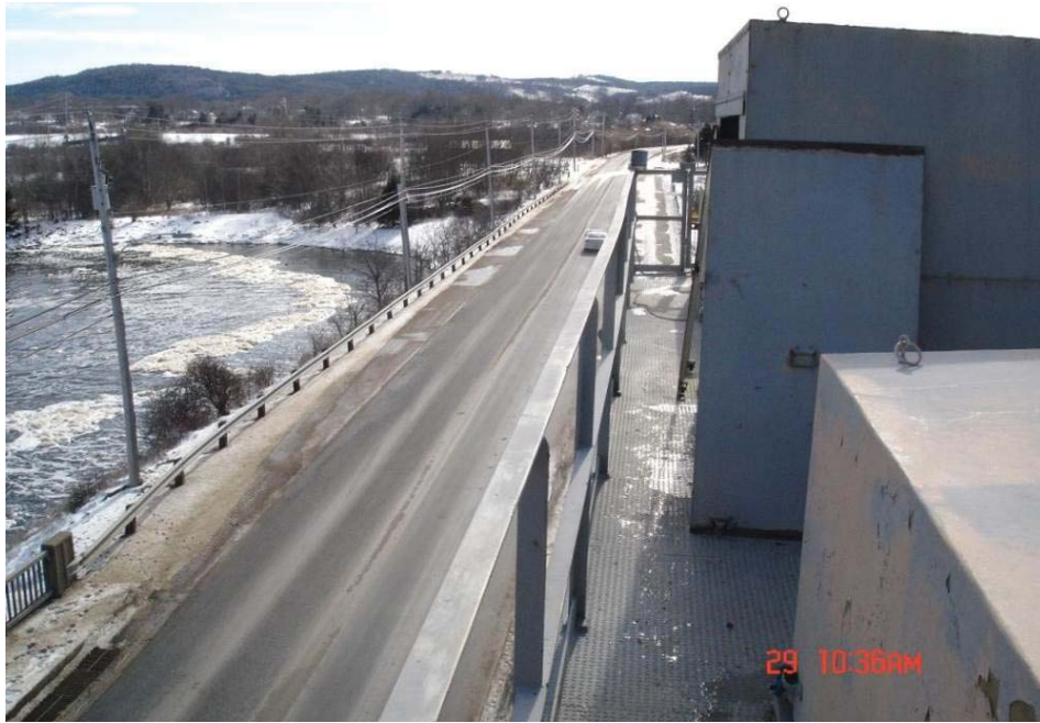
Photo 14 – Hoist Assembly Enclosures
