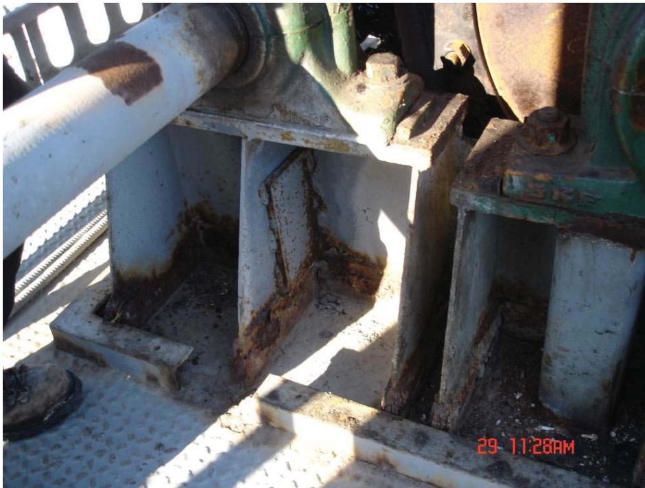
Photo 5 – Reinforced Rope Drum Support Stiffeners
