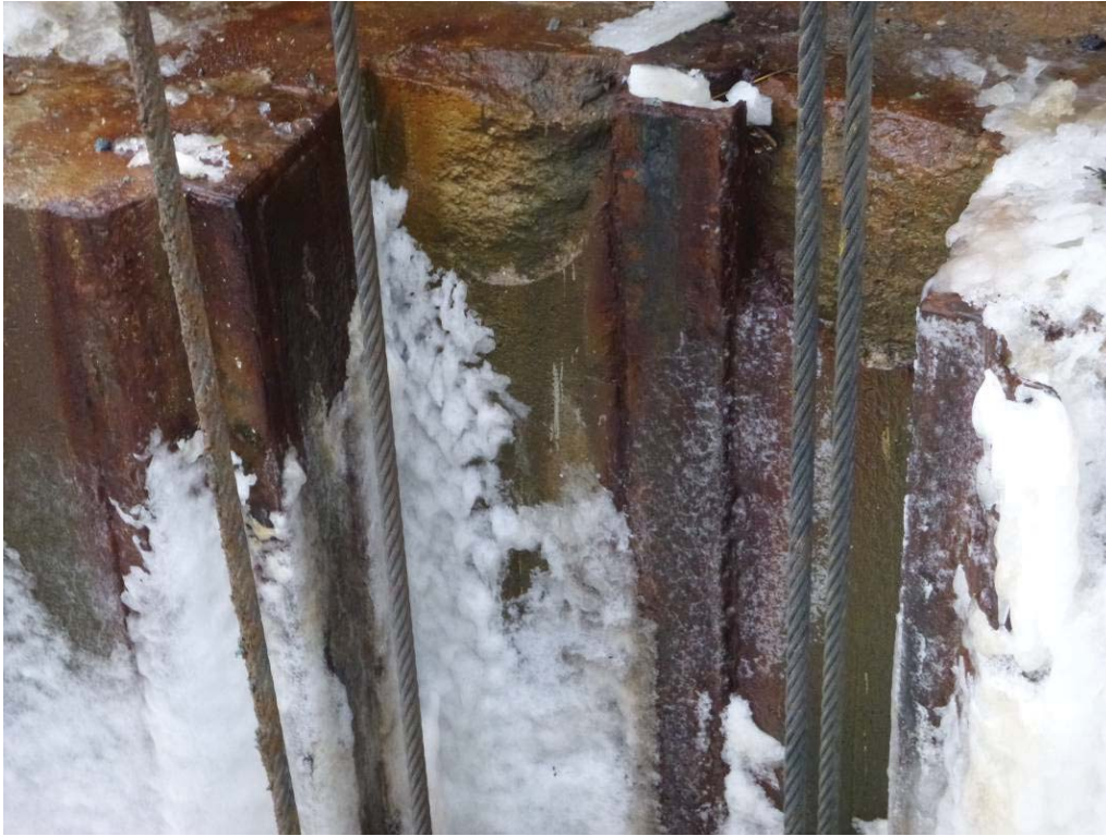
Photo 7 – Gate Side Guide (Top), Corrosion, Concrete Spalling
