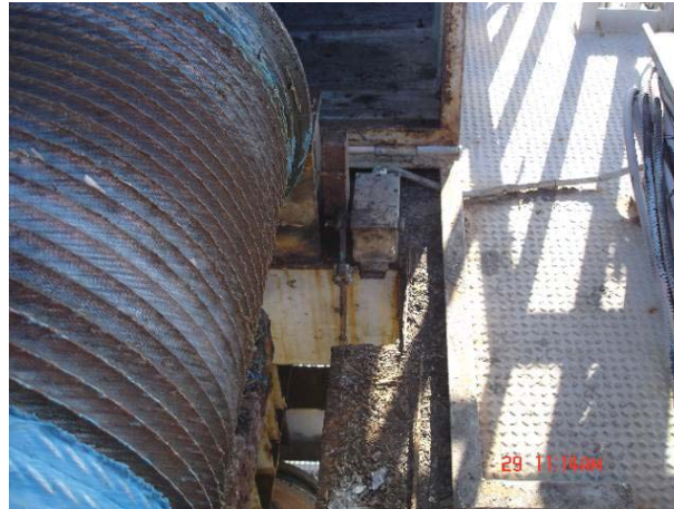
Photo 23 – Drum Enclosure Severe Deck Corrosion
