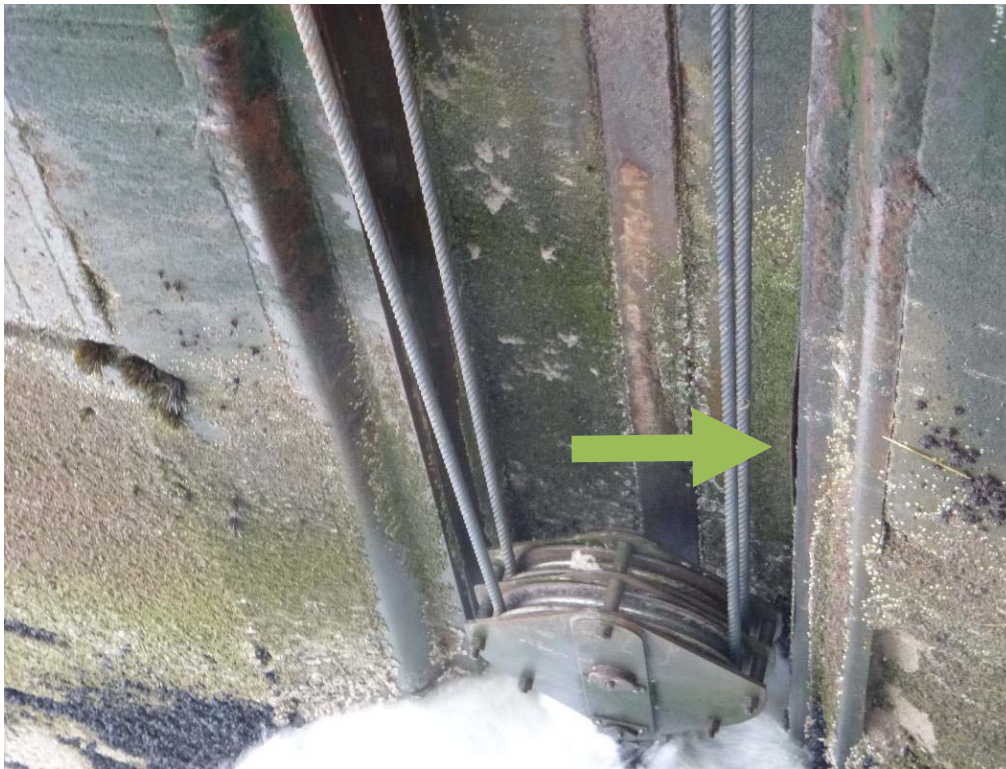
Photo 8 – ¼” Roller Path Overlay Plate Separation
