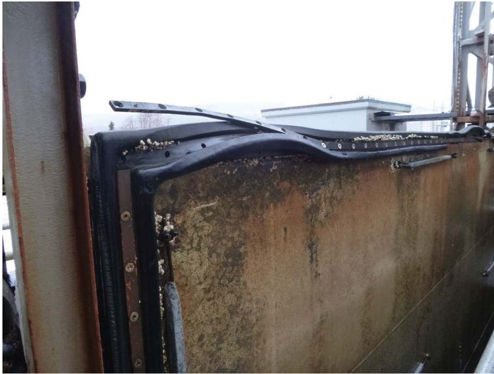
Photo 9 – Damaged Lintel Seal on Spillway Gate #2
