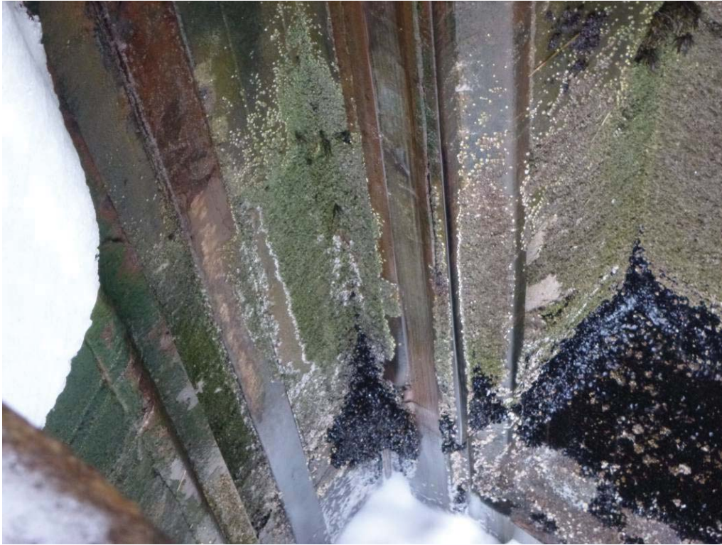
Photo 11 – Deformed ¼” Overlay Plate (Reservoir Side)
