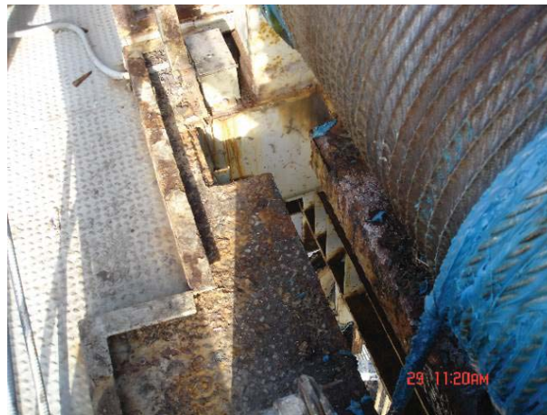
Photo 24 – Drum Enclosure Deck Penetration
