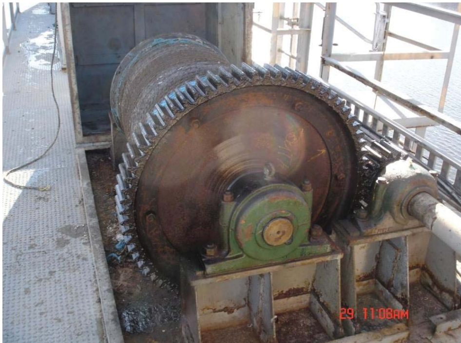
Photo 16 – Unguarded Rotating Drum Components
