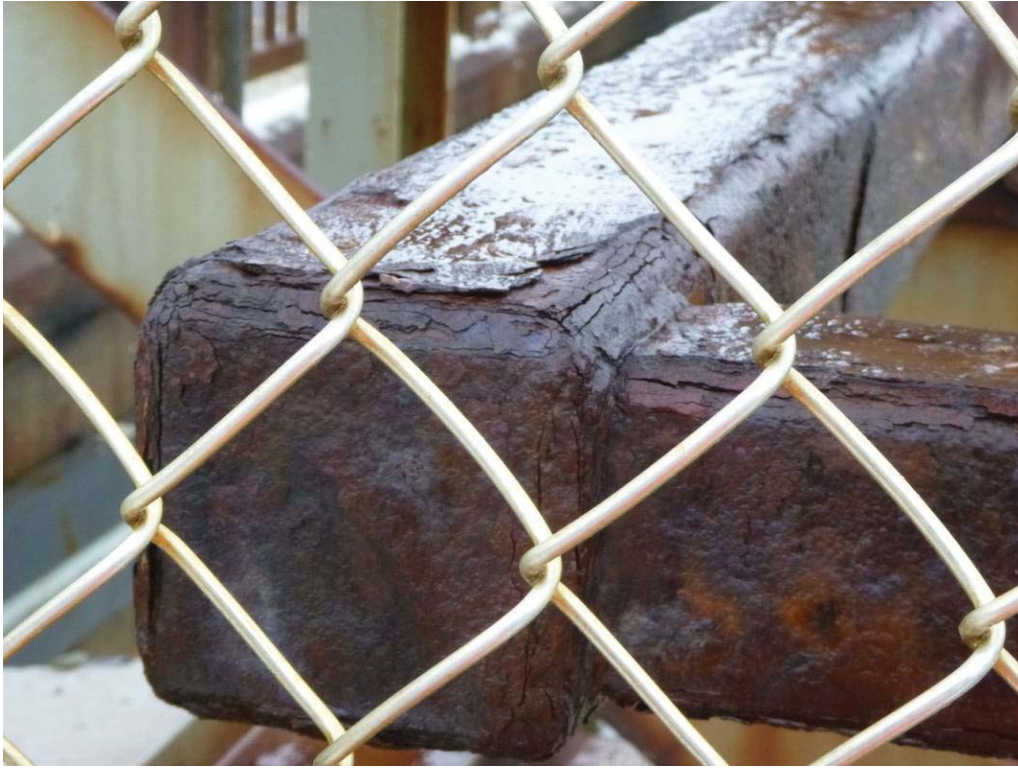
Photo 3 – End Ladder Support L-Bracket Severe Corrosion
