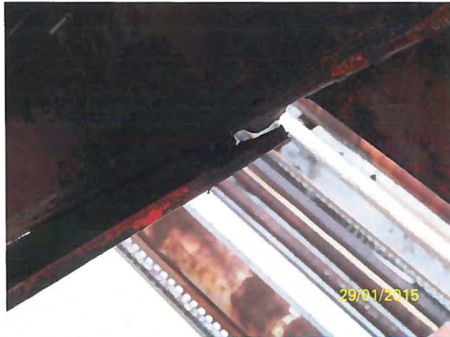
Photo 10 - Deteriorated Connection between Batten Plate and Channel
