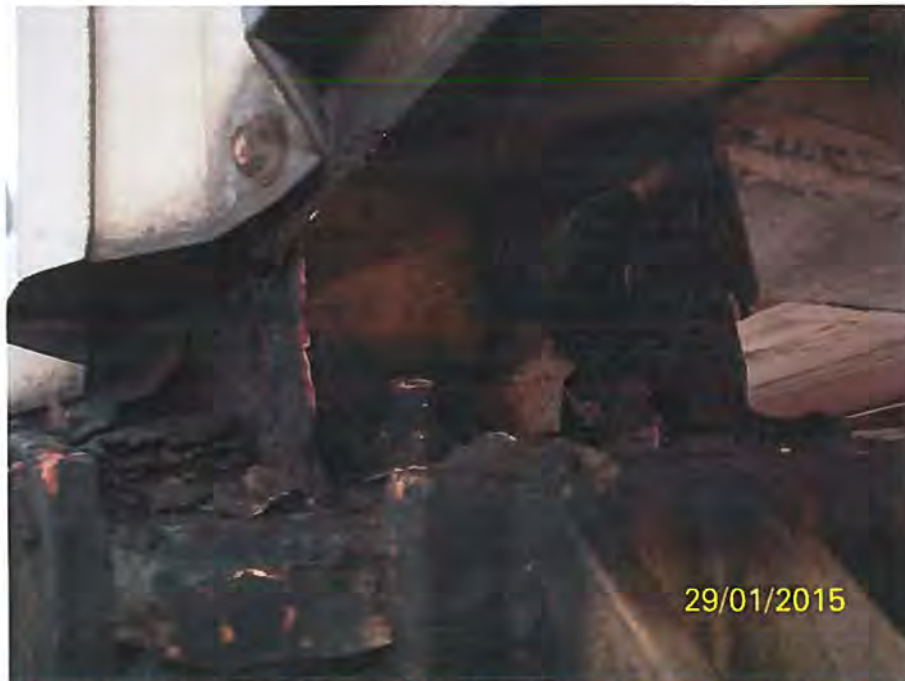
Photo 1a - Deteriorated Flanges at West Side Bearing, Viewed from the North
