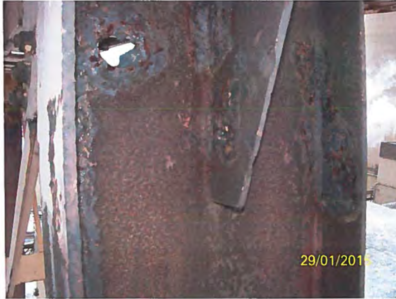
Photo 3a - Hole through the web of the W18x45 Column just below the West Bearing
