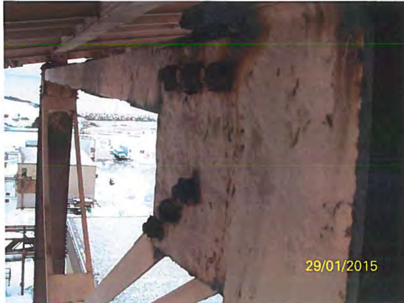
Photo 5a - Deteriorated Gusset Plate
