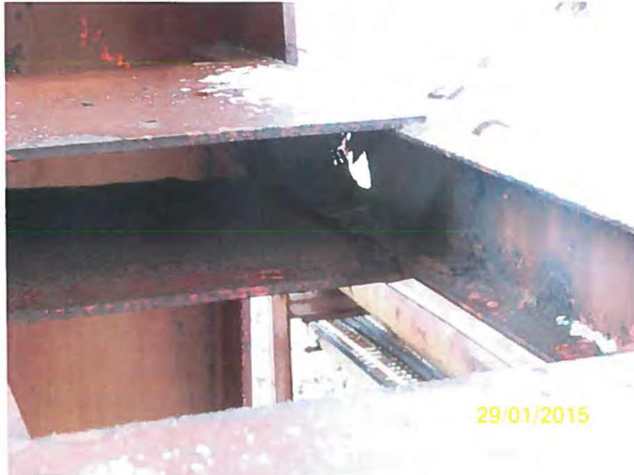
Photo 10a - Holes through web and Flange of Channel Making up Lower Horizontal Strut
