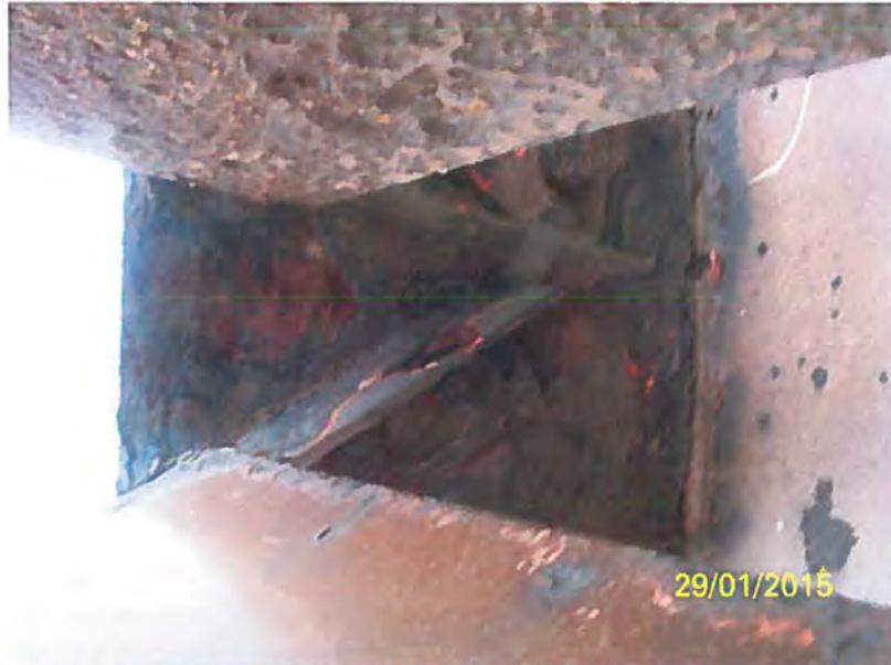
Photo 7a - Deteriorated Gusset Plate, Corroded Angle and Channel Sections
