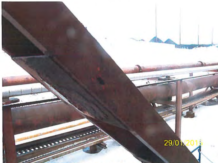
Photo 11a- Holes through the web of the lower diagonal Strut
