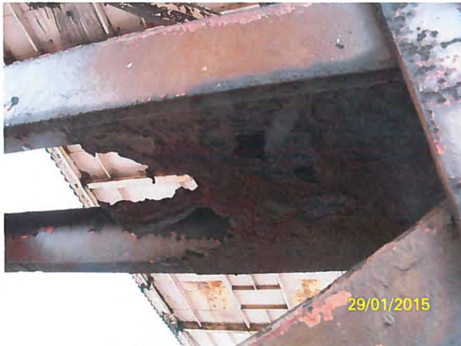
Photo 8a - Deteriorated Batten Plate
