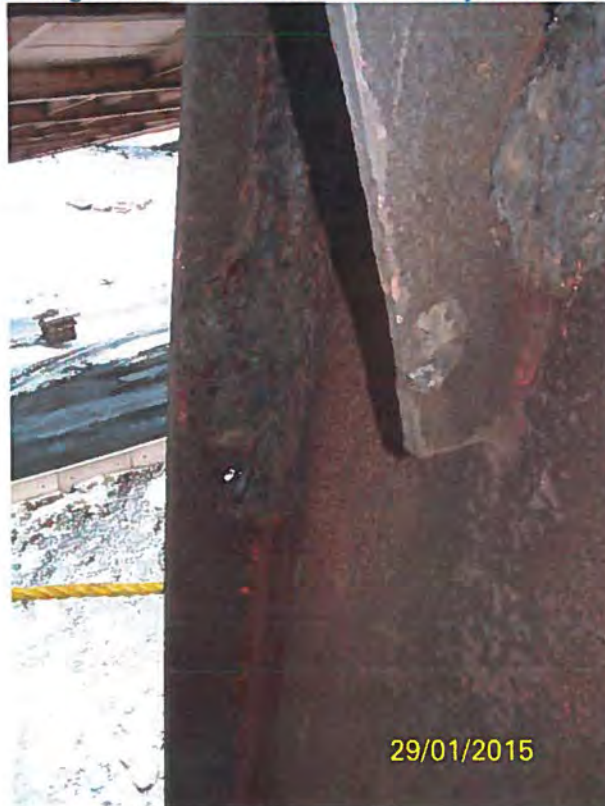
Photo 3b - Hole through the Flange of the W18x45 Column just below the West Bearing
