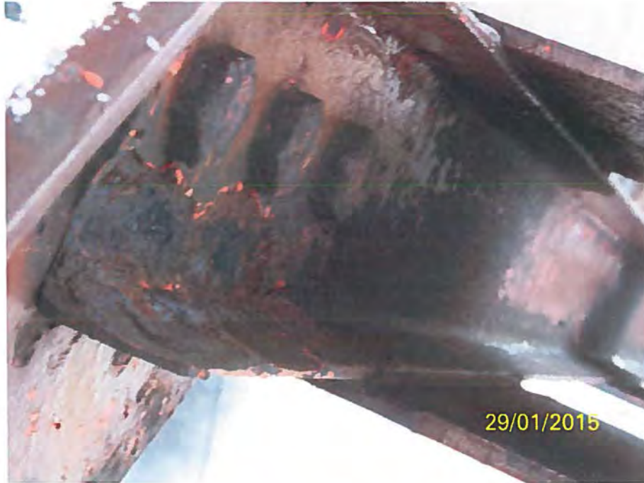
Photo 9 - Corrosion on the web and Flange of Diagonal Strut
