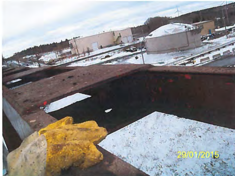
Photo 6a - Hole through Batten Plate
