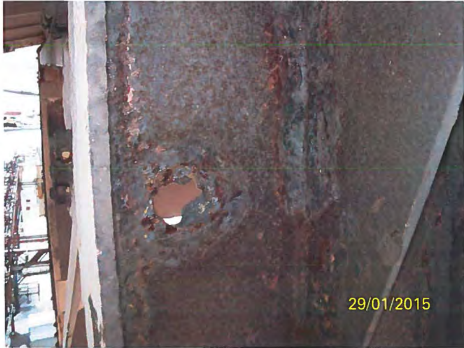
Photo 3c - Another View of holes through web and stiffener
