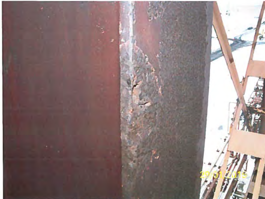
Photo 4a - Pitting in Flange of W18x45
