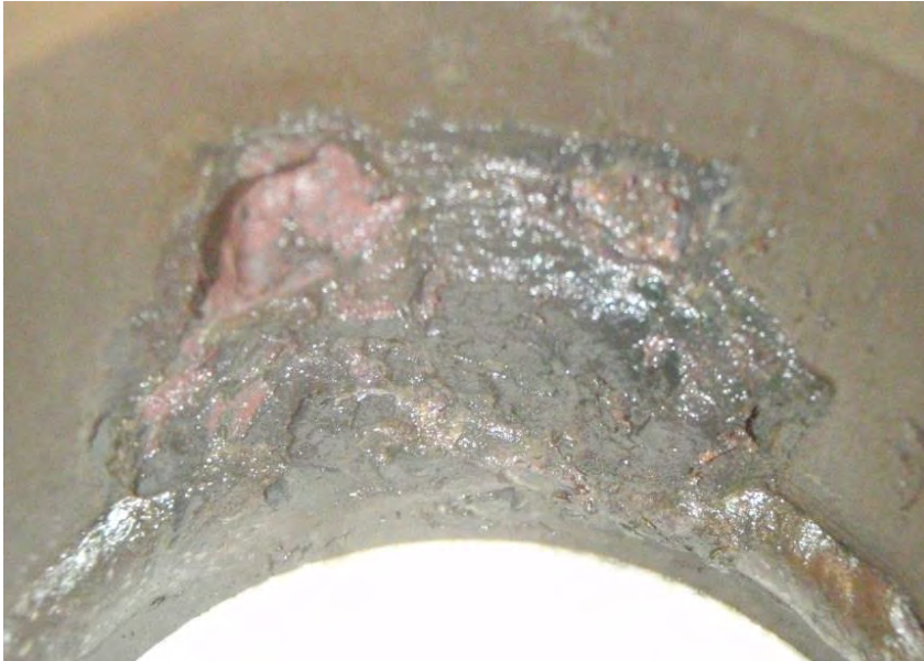
Photograph 17 3 rd Stage at 24 Hours: Second EDTA at 24 Hours (or 48 hours total in Iron Oxide Removal Stage), Hot Side
