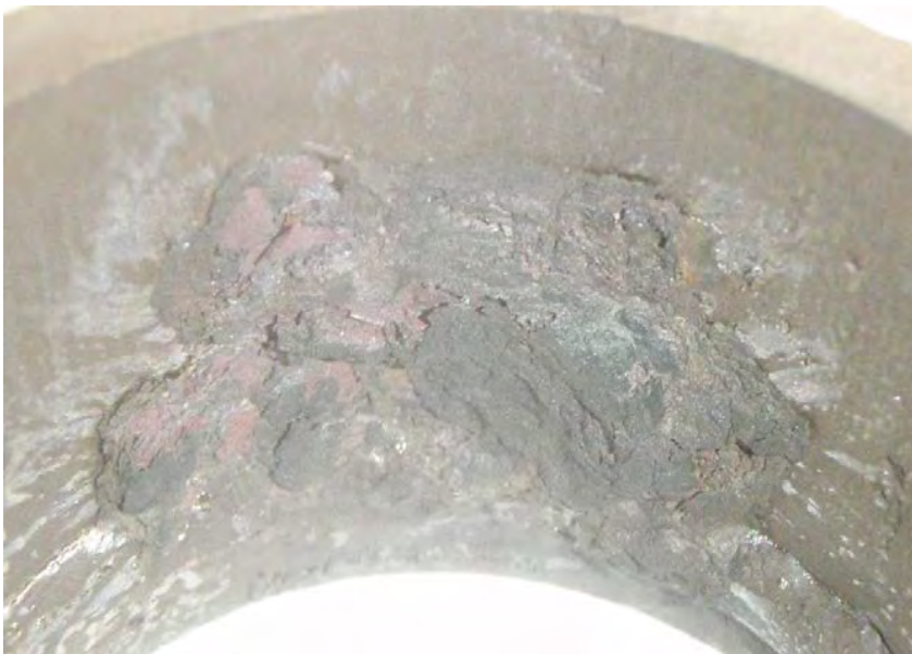
Photograph 18 End of 3rd Solvent Stage (45.3 hours in 2 nd Batch of EDTA) Iron Oxide Removal Stage (at ~69-70 Hours Total Contact)
