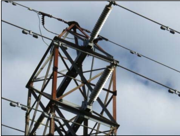
Ph 1 – Corroded tower members (1 of 3).
