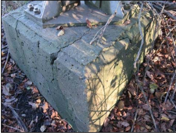
Ph 1 – Foundation cracks (1 of 3).
