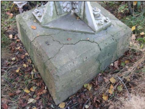
Ph 3 – Foundation cracks (3 of 3).
