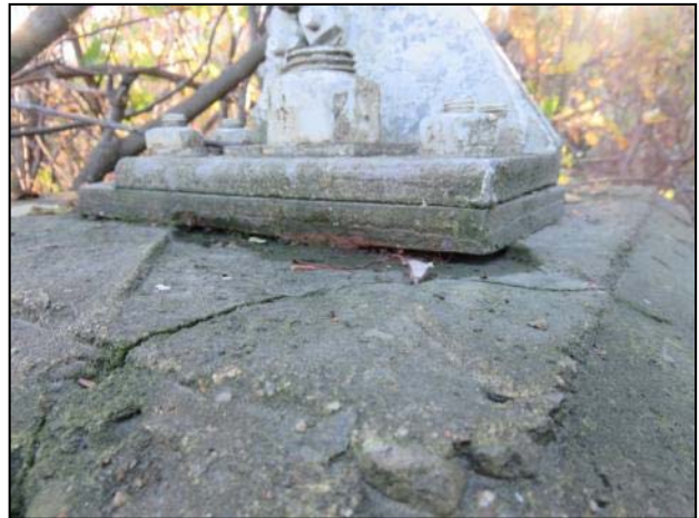
Ph 4 – Gap beneath base plate.
