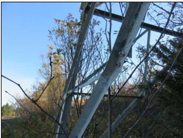
Ph 5 – Bent tower diagonal (2 places).
