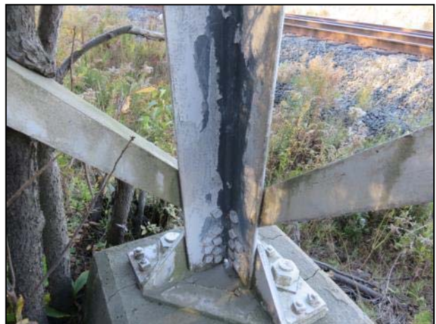
Ph 6 – Paint condition (typ.).
