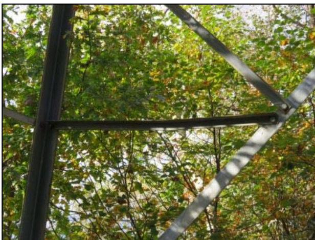
Ph 5 – Bent tower member.
