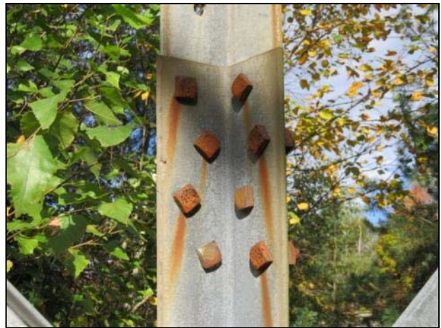
Ph 4 – Corroded bolts (typ.)..
