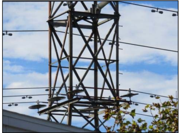
Ph 2 – Corroded tower members (2 of 3).
