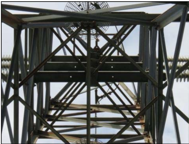
Ph 3 – Corroded tower members (3 of 3).
