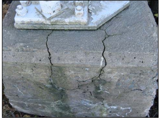
Ph 2 – Foundation cracks (2 of 3).
