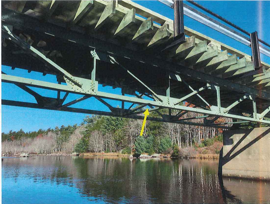
Photo 17 - MINOR DENT IN BOTTOM CHORD OF 3RD TRUSS FROM W
