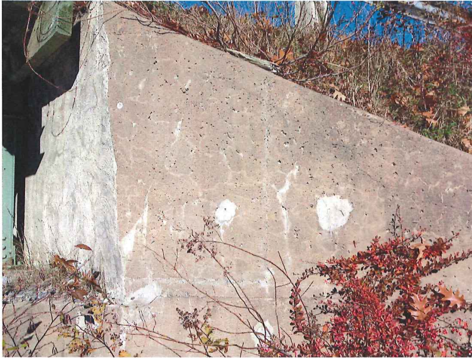
Photo 7 - SE WINGWALL, SOME PATCHING
