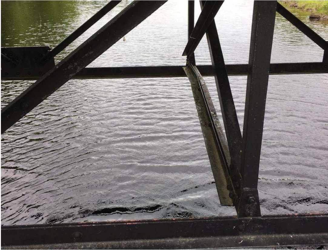
Photo 11 - DEFORMED BOTTOM CHORD OF WEST DIAPHRAGM BRACE
