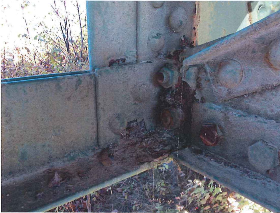
Photo 15 - CORROSION AT PANEL POINT, TYPICAL AT E END OF E SPAN
