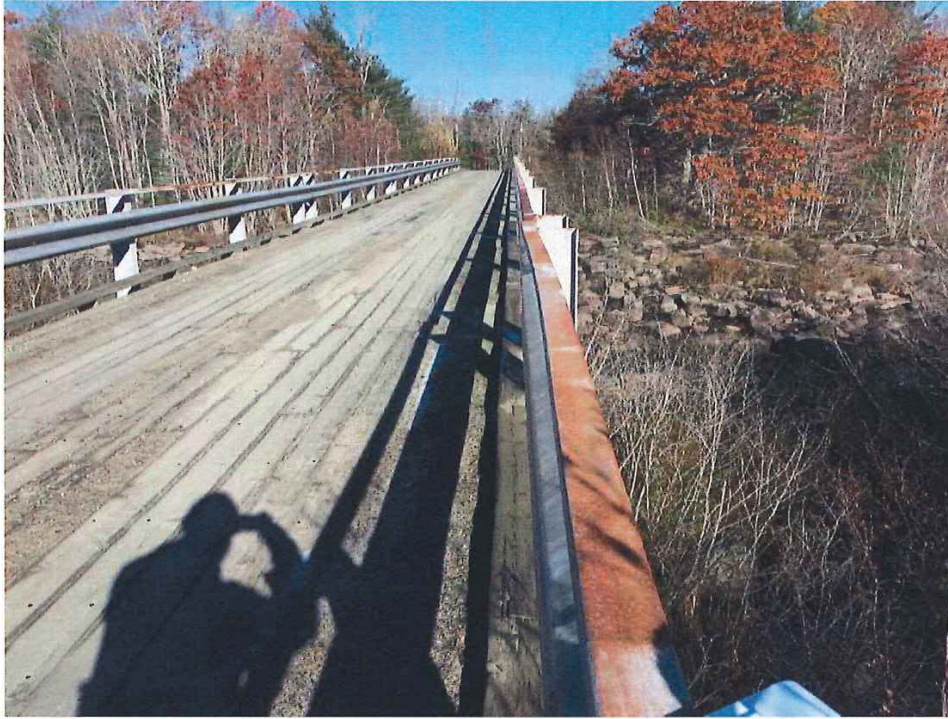
Photo 3 - MINOR BEND IN SE BRIDGE RAIL
