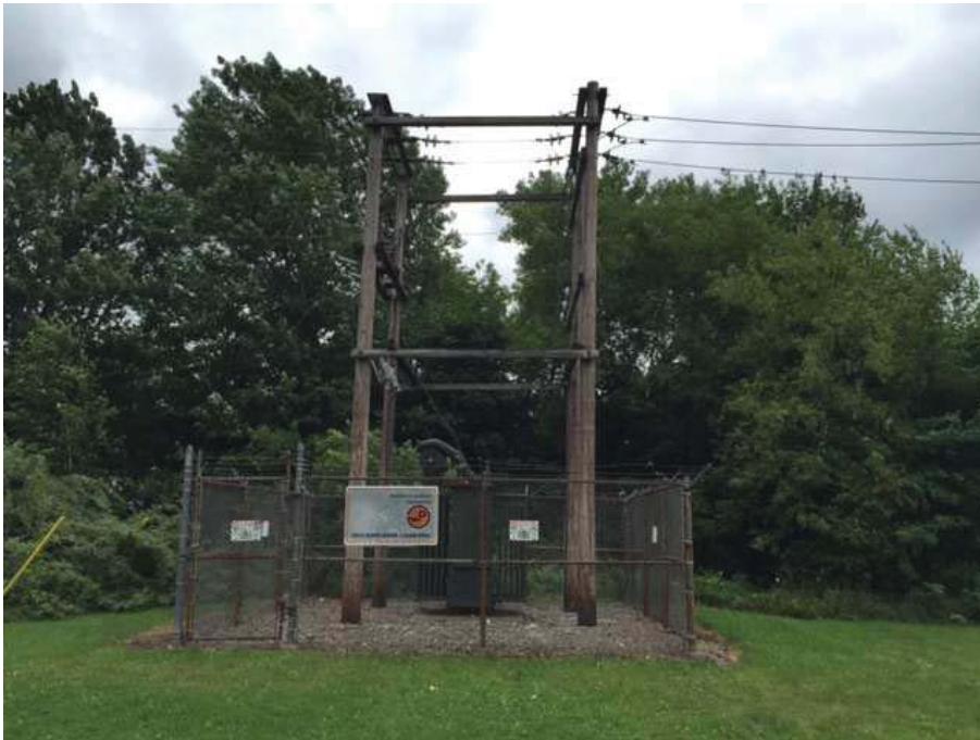
Figure 11 Photo of 534N-Duchess Ave
