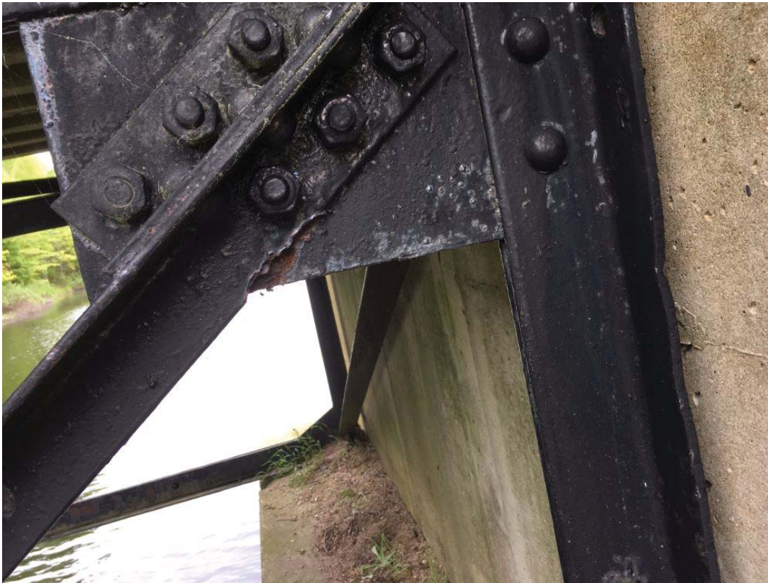
Photo 12 - TYPICAL PACK RUST AT CONNECTIONS
