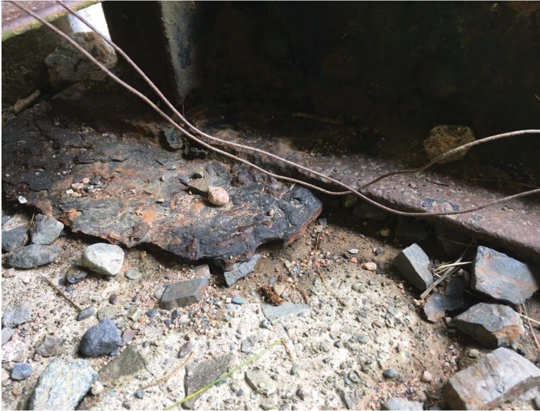
Photo 13 - SEVERE SECTION LOSS AT NW TRUSS BEARING PLATE
