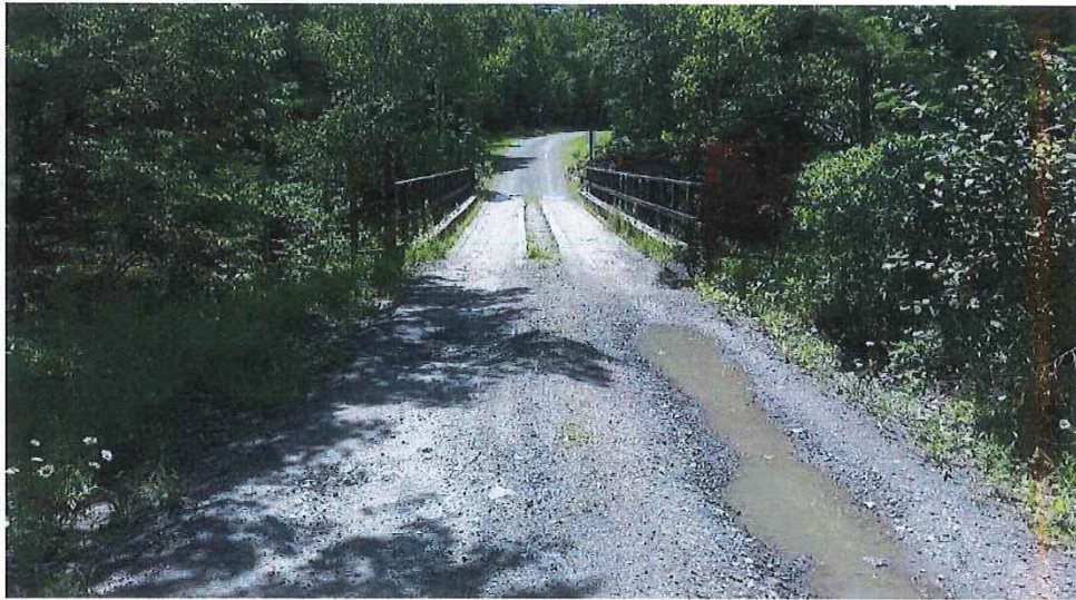
Photo 1 - North Approach Looking South - Rut and Edge Erosion
