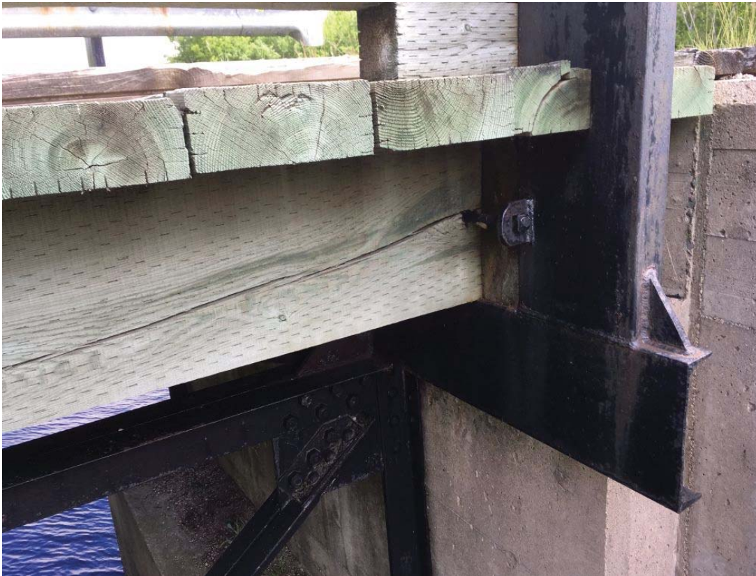
Photo 13 - SPLIT TIMBER BEAM AT SE CORNER GUARDRAIL CONNECTION
