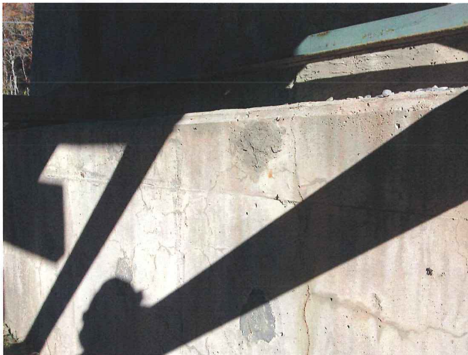
Photo 8 - W BREASTWALL/BEARING SEAT
