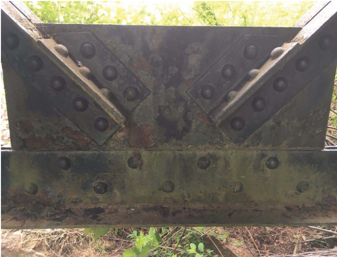
Photo 11 - TYPICAL COATING FAILURE AND CORROSION AT CONNECTIONS
