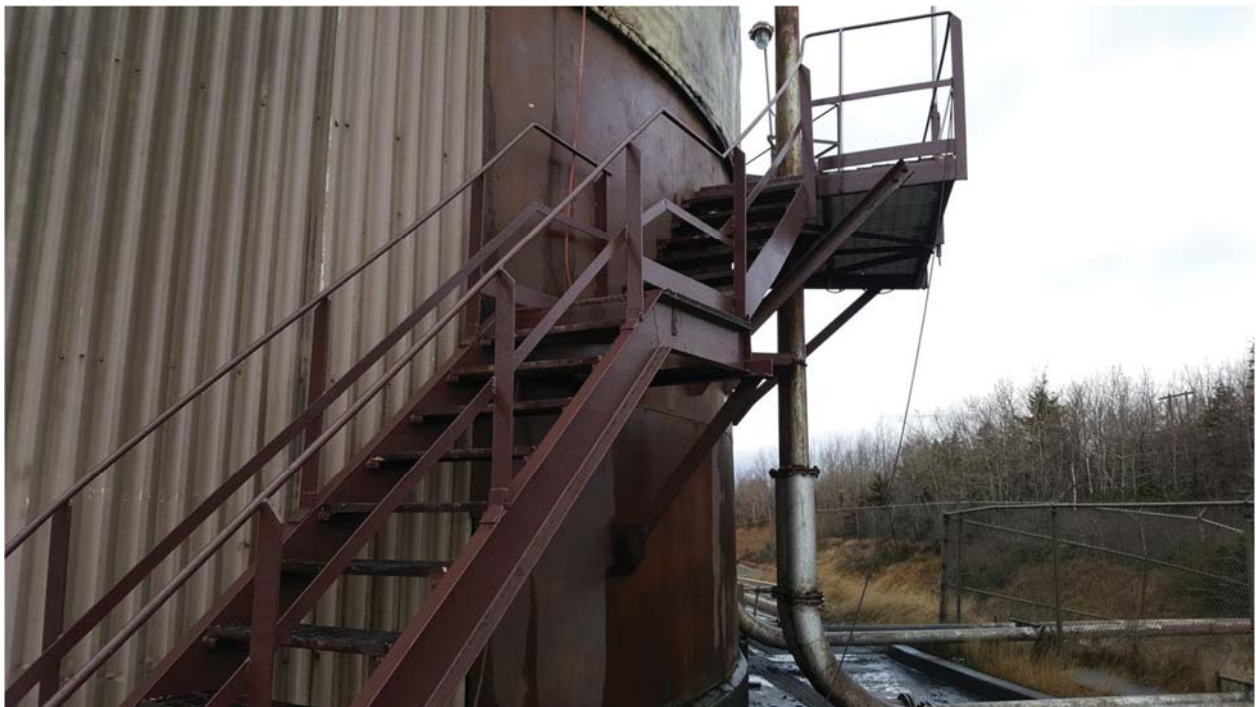
Photo 2: Showing a view of the first two stair run (from ground elevation).
