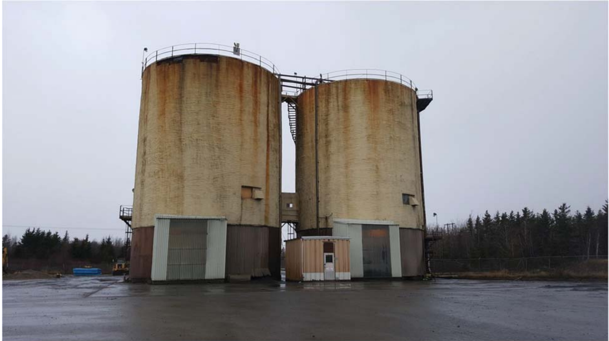
Photo 1: Showing a view of the Ash Silos – Stair System runs along the back side of the North (right) Silo.
