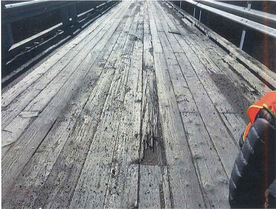
Photo 5 - TYPICAL DECK - WORN AND PUNKY IN SPOTS. LOOSE SPIKES.
