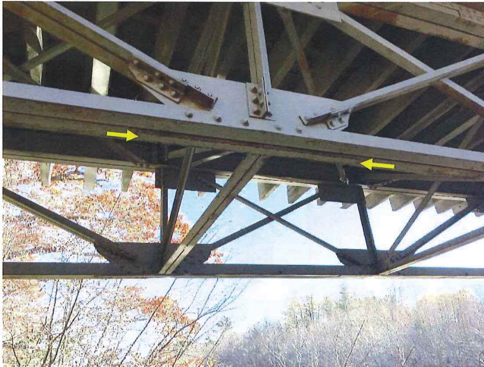
Photo 11 - PLATE WELDED ON BOTTOM CHORD IN SEVERAL LOCATIONS
