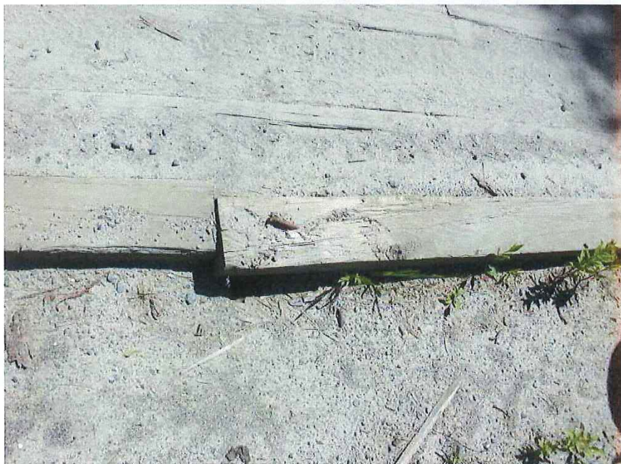
Photo 6 - Nails sticking out of wearing surface
