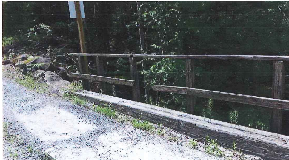
Photo 4 - Railing broken at S/W corner
