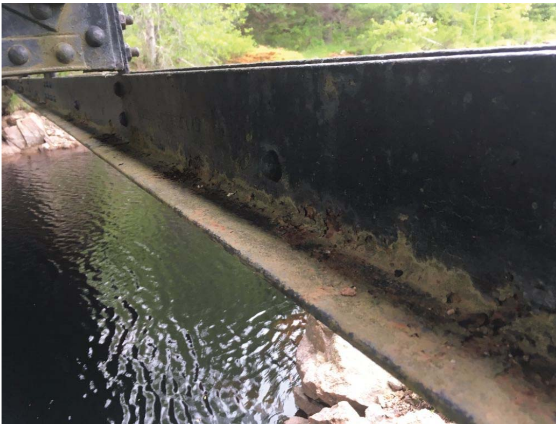
Photo 12 - CORROSION ON TOP SURFACE OF BOTTOM TRUSS CHORD
