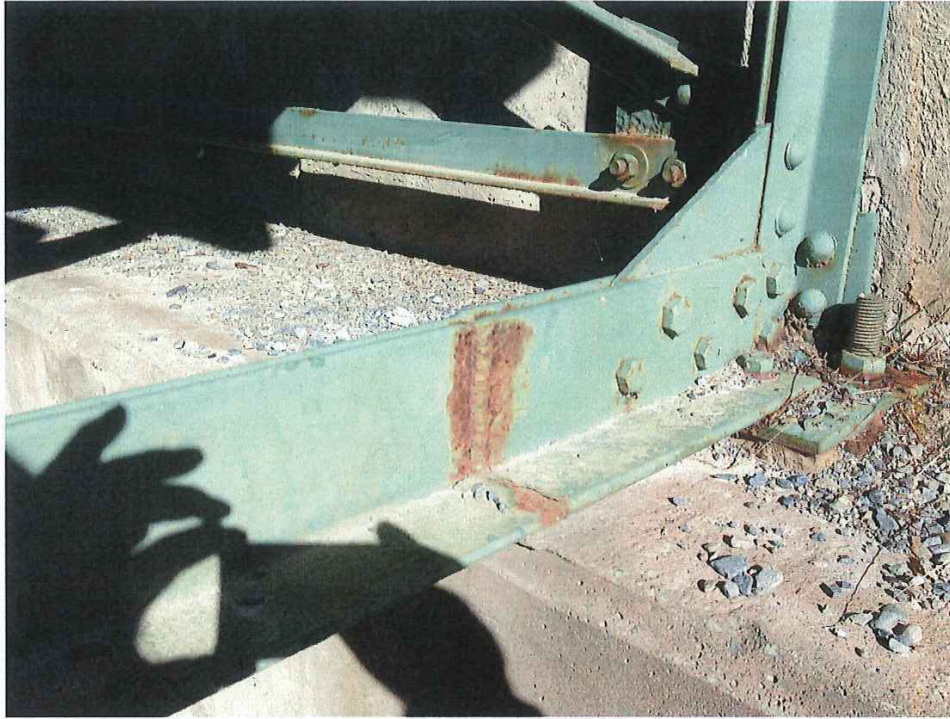
Photo 9 - PAST REPAIR TO BOT CHORD, SE BEARING ON E SPAN
