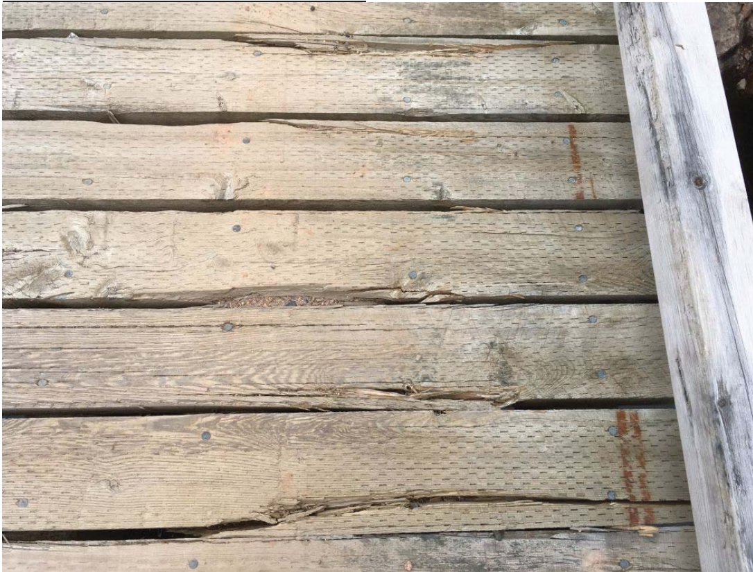
Photo 9 - EDGES OF DECK TIMBERS SPLIT (TRACKED MACHINE DAMAGE)
