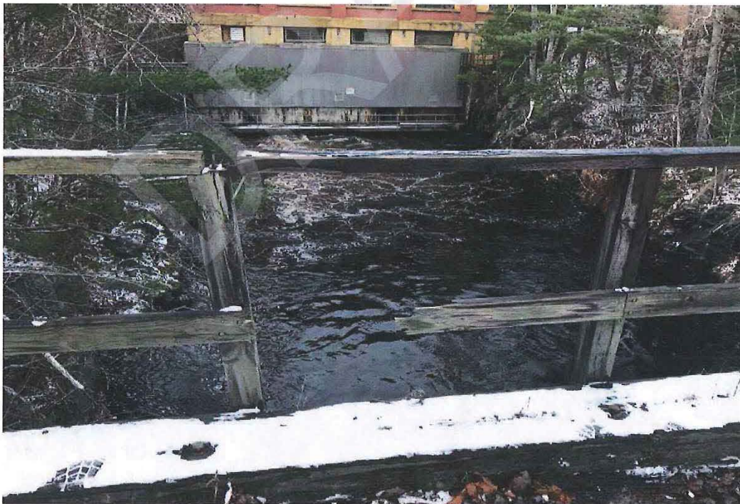
Photo No. 4 – Damaged Guard Rail
