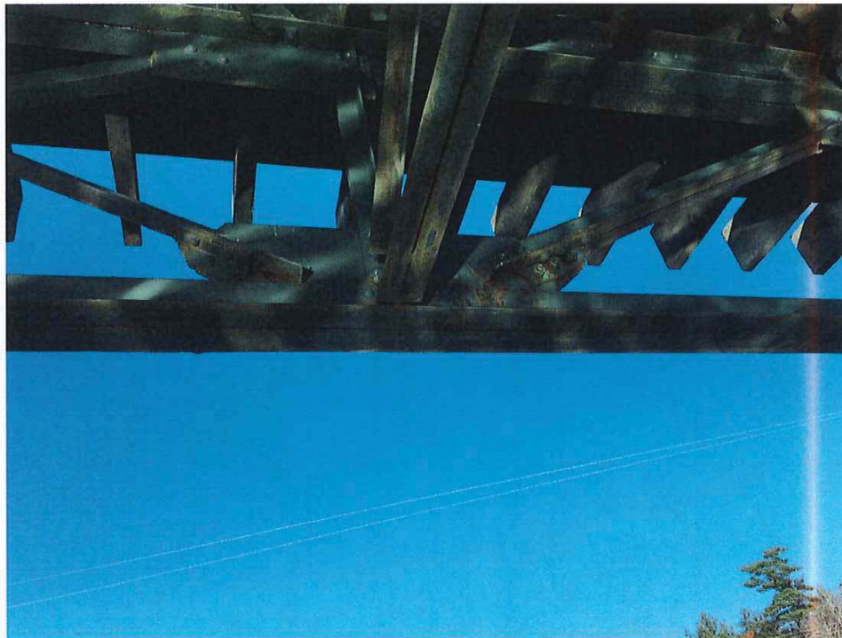
Photo 18 - TYPICAL PANEL POINT, MINOR CORROSION
