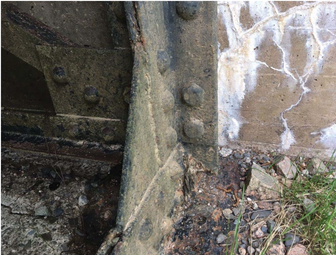
Photo 14 - SEVERE SECTION LOSS AT NW TRUSS BEARING VERTICAL
