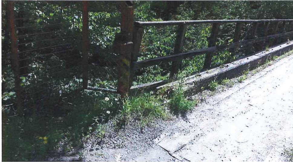
Photo 7 - Wheel Guard and railing broken at N/E corner
