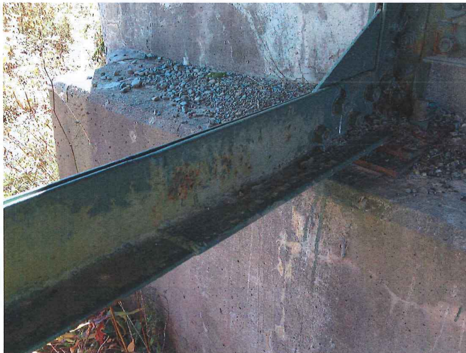
Photo 20 - PAST REPAIR TO SW BOT CHORD AT BEARING
