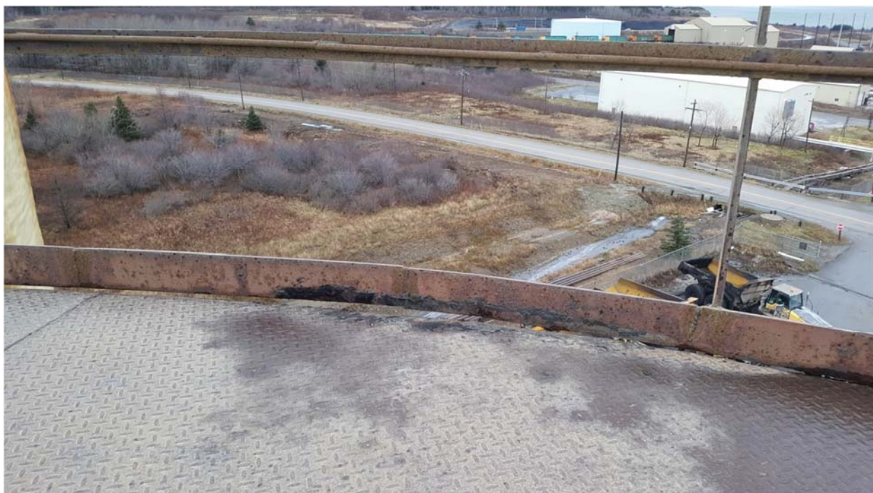
Photo 5: Showing a view of the Ash Silo roof kick plate with minor corrosion present.
