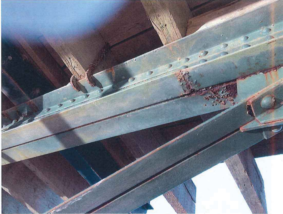
Photo 13 - APPARENT REPAIR TO BOT FLANGE OF TOP CHORD, E SPAN
