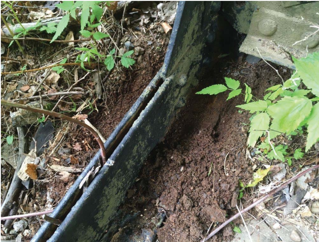
Photo 10 - TRUSS BEARINGS BURRIED IN DEBRIS AT E ABUTMENT
