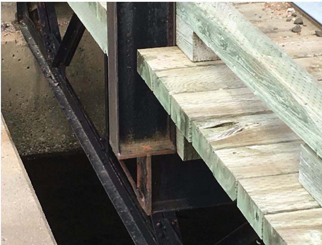
Photo 14 - WEAK STIFFENER DETAIL AT GUARD TO DECK BEAM CONNECTION
