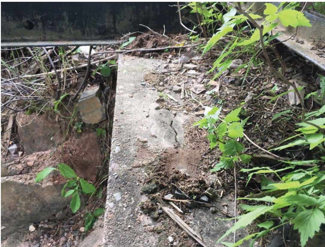
Photo 16 - LONGITUDINAL CRACK ON TOP OF E ABUTMENT
