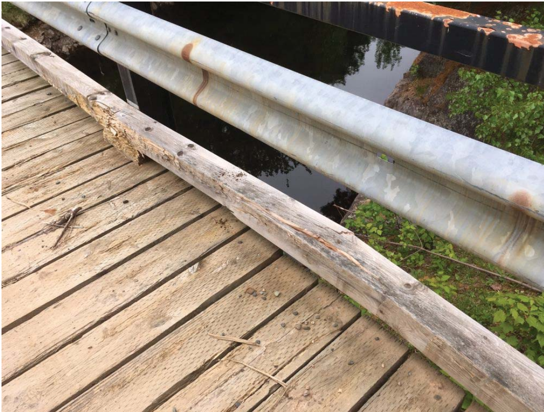
Photo 8 - BROKEN WHEEL GUARD SW CORNER
