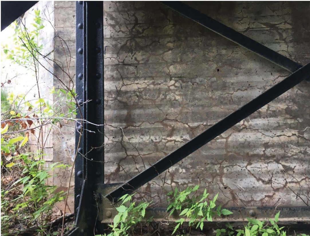
Photo 17 - E ABUTMENT MAP CRACKING IN BACKWALL
