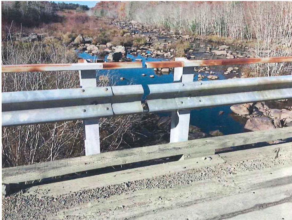
Photo 4 - TYPICAL "EXPANSION JOINT"
