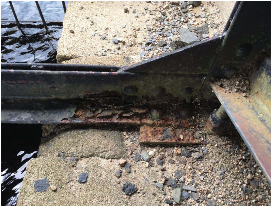
Photo 9 - SECTION LOSS AT SW TRUSS BEARING
