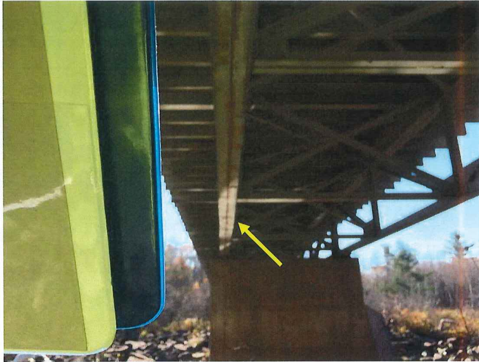
Photo 9 - LOOKING AT MINOR BEND IN E BOT CHORD OF N TRUSS
