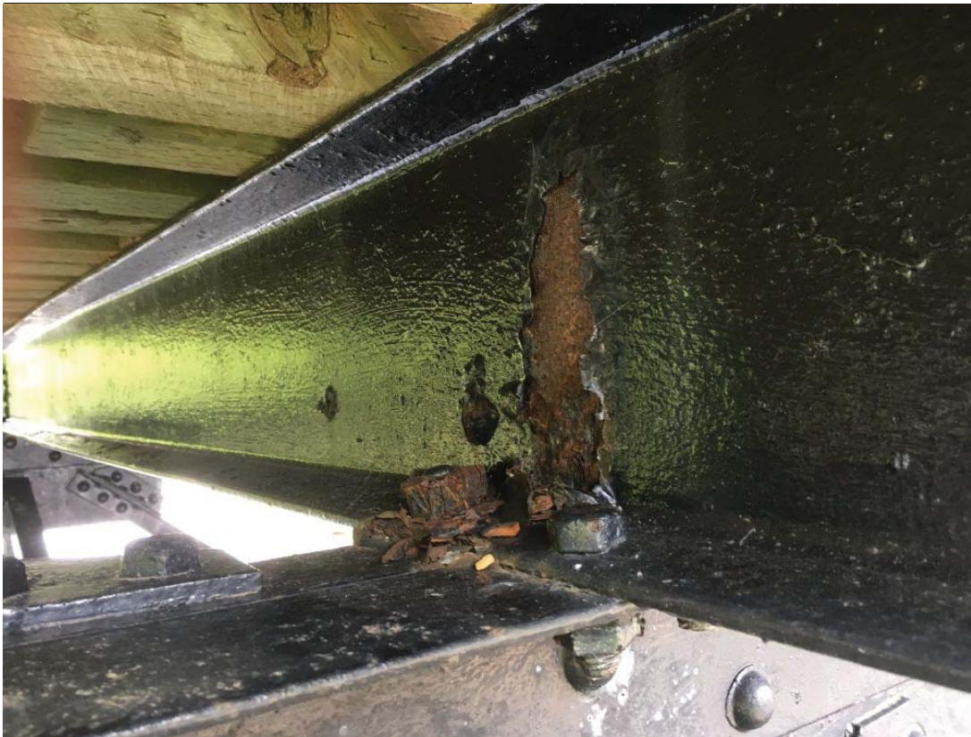
Photo 10 - TYP. CORROSION ON DECK BEAMS OPPOSITE BEARING STIFFENERS
