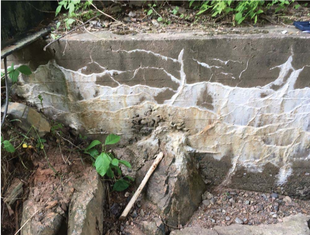
Photo 15 - E ABUTMENT CRACKING, EFFLORESCENCE, AND SEGREGATION
