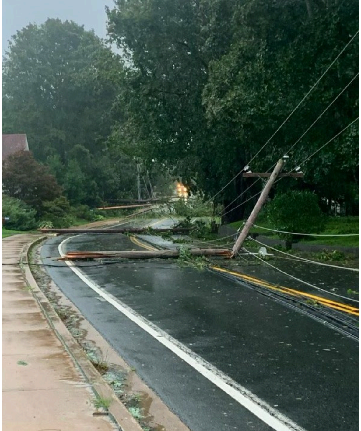
Figure 69 - Broken Distribution Poles during Post Tropical Storm Lee
